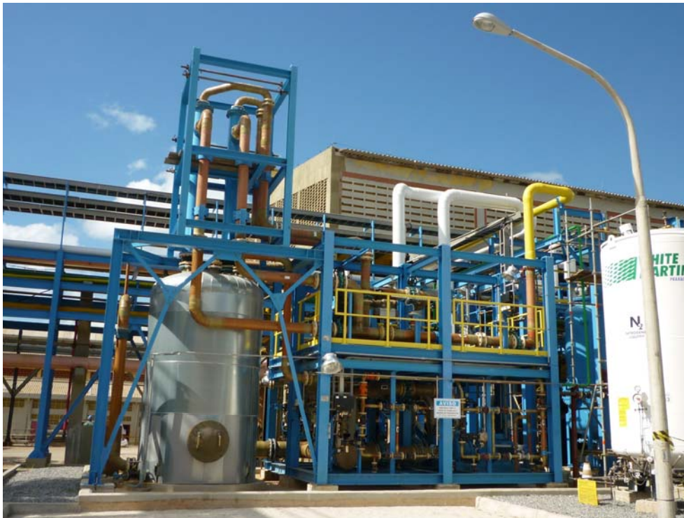
The hypochlorite module supplied by tkUCE Italia Sodium Hypochlorite Production
